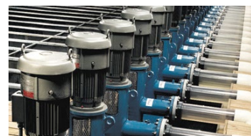
Vertical Pump in Operation
