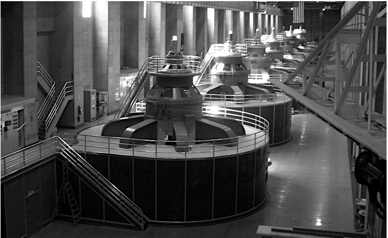
DMX® application - Flovel India hydro turbine main guide bearing
